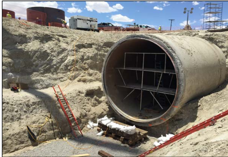
PHOTO: Contractors continue to make progress on the replacement of the 40-foot portion of the pipe on May 30, 2016 (Photo courtesy of the Bureau of Reclamation).
