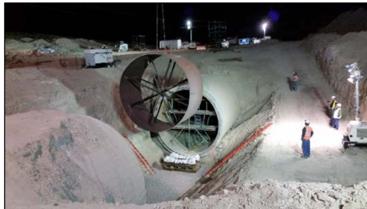
Photo: The first section of pipe being lowered into place at the breach site on May 29, 2016 (Photo courtesy of the Bureau of Reclamation).
