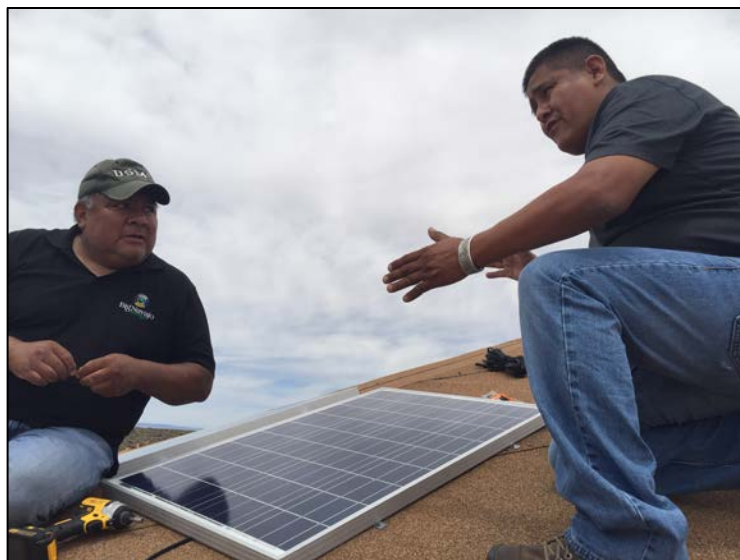
PHOTO: Council Delegate Otto Tso (right) and Big Navajo Energy president Dory Peters (left) install solar panels on the home of Lloyd Billy near the community of Tuba City, Ariz.
