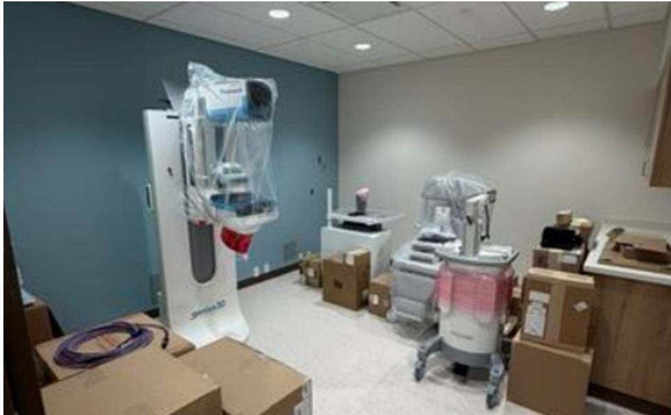
Mammography Equipment Installation
