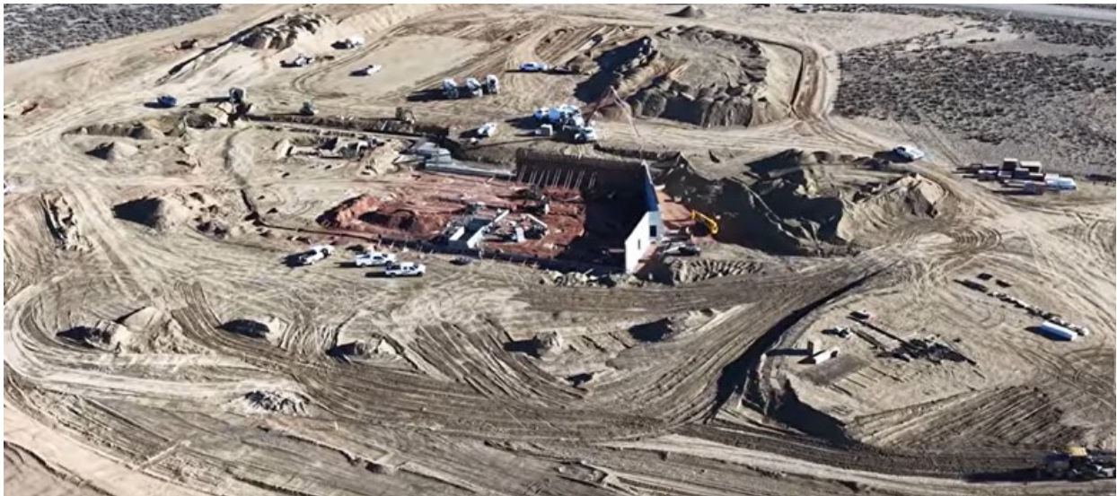
Site Drone Photo of the Civil Work at Pueblo Pintado Healthcare Facility
